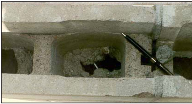
Figure 2 - Mortar droppings on truss-type joint reinforcement diagonal cross-wires
